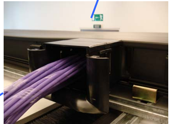
Providing safe radius on exiting UTP
